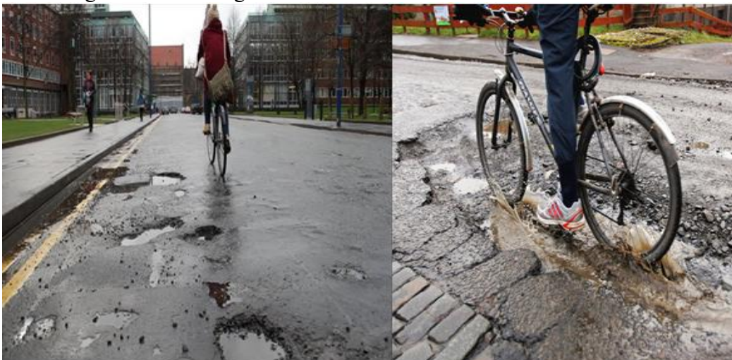
Figure 2.2. Damage to the road surface.
